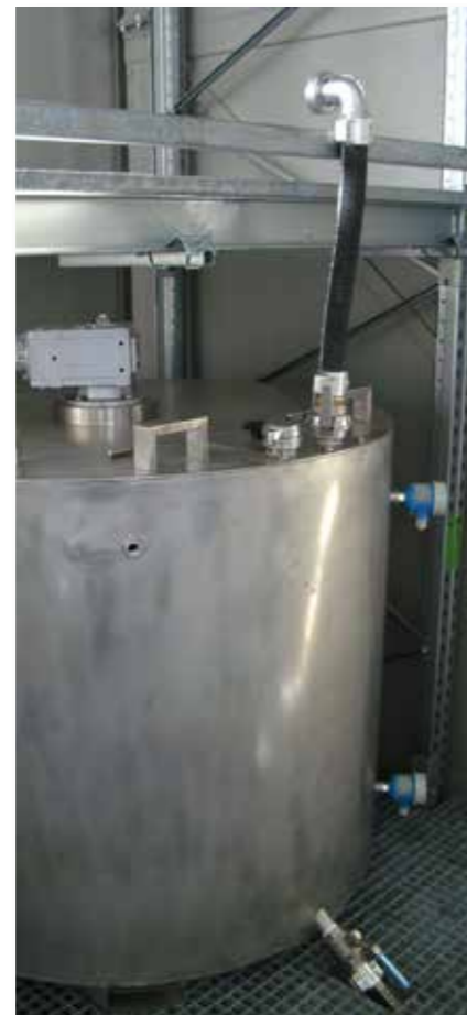
Resin tank and mixer
